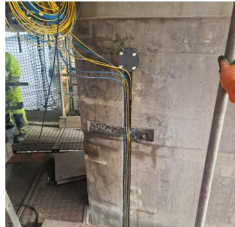
Reference electrode installed with associated wiring
