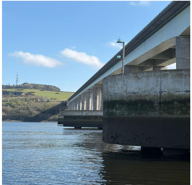
Bridge Pontoons showing green, yellow and red marker lights at navigation channel
